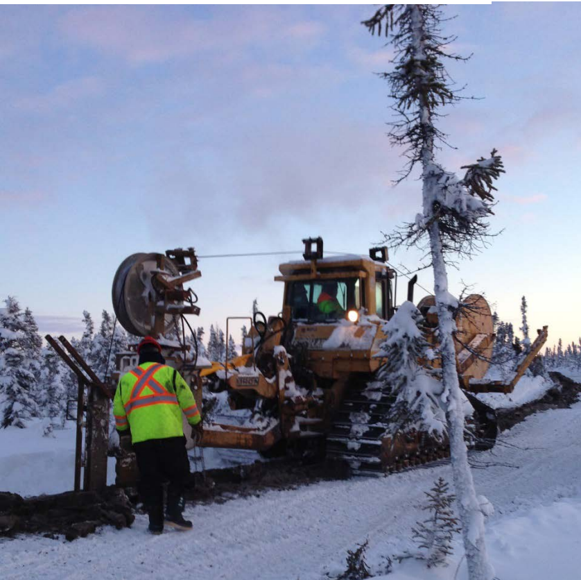
Quality assurance review of the cable plough installation on the wilderness segment of the build.
