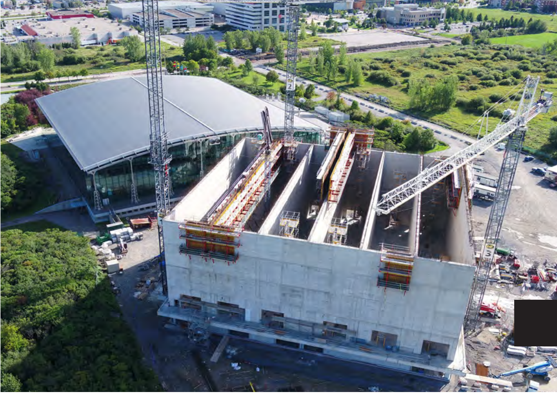
Construction progress at the site in April 2020, in the midst of the pandemic.
